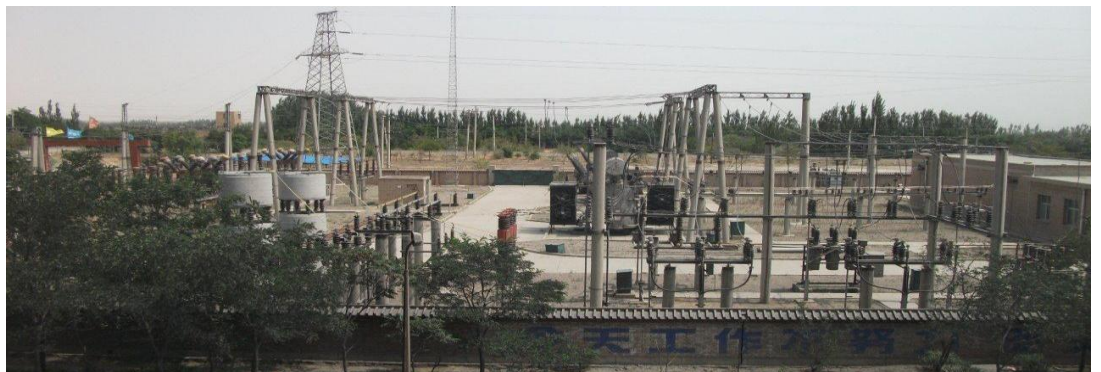
Electricity Sub Station
